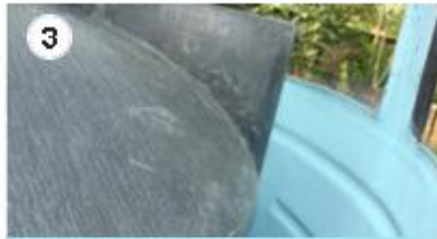
3 The fermentation tank has an outer water jacket that circulates solar heated water to maintain an ideal temperature for working of anaerobic bacteria.
