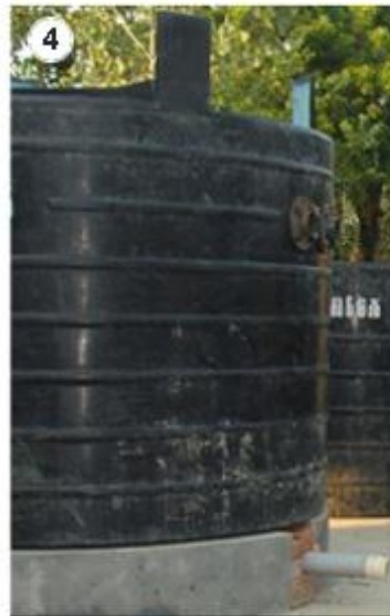
4 The manure in the fermentation tank gets stirred by a pump to avoid settlement, and for thorough decomposition. The decomposing manure then produces biogas, which is moved to the gas holder tank.
