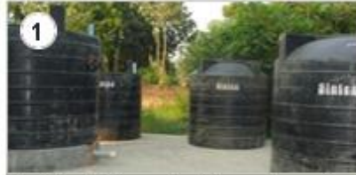
1 The Model Biogas Plant is a set up with four tanks, placed over ground. This enables temperature control in the system for steady production of biogas all year round.
