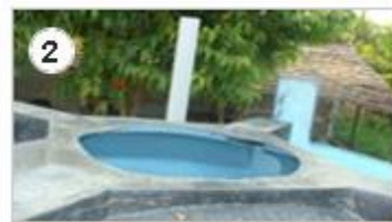
2 The first tank is the fermentation tank. Cattle manure is fed into it through an inlet.
